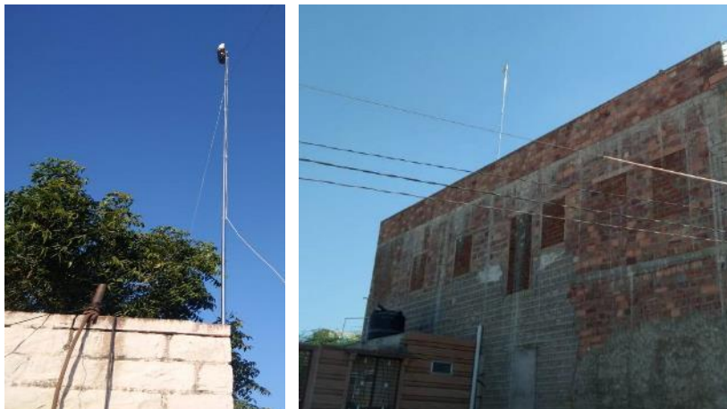
Picture - Access Points for Intranet Connectivity installed at suitable locations
